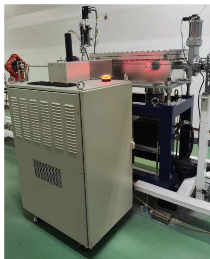
Figure 9: Kicker magnet and its high stability pulsed power supply installed in the undulator tunnel.
